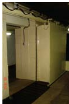
Radiation Shielding door in Mat.Sc.-II
