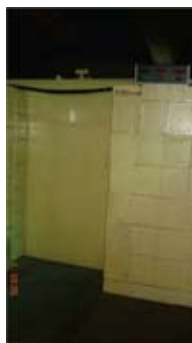
Radiation shielding door in HYRA, BH-II
