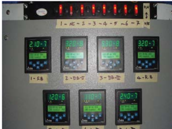
Fig. 3: Vacuum interlocking Gauges for LINAC area
