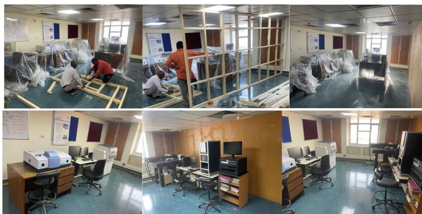
Figure 4.13: Various pictures of the progress of the dark room, which is almost complete in the CCMC area for performing the UV photoluminescence and solar simulation measurements.
