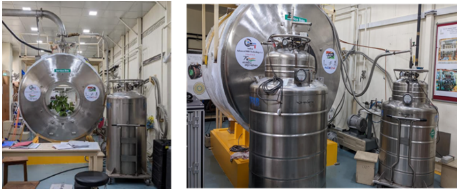
Figure 3.9: (a) The precooling of the MRI magnet using LN2 is in progress, (b) the cooling of the MRI magnet using LHe is in progress.
