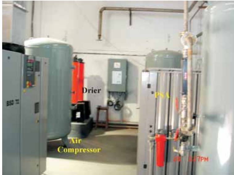
Fig.3. New PSA system of upgraded LN2 Plant
