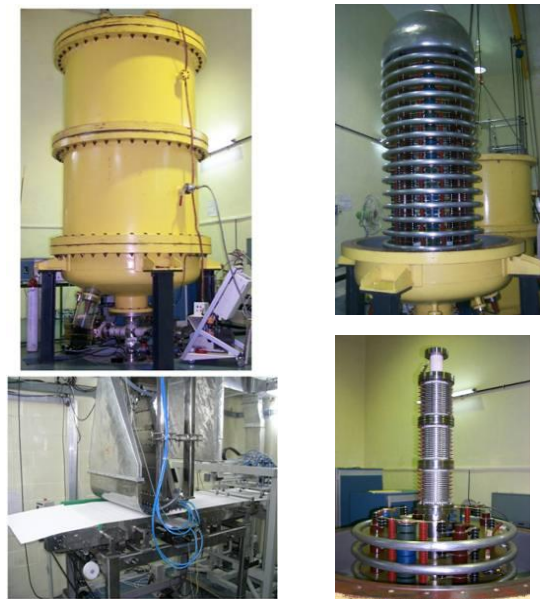
Figure 1. The DC accelerator (left), HV assembly (right top), gun & acceleration column (right bottom).
