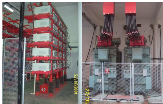
Figure 5: RHVPS and multi secondary transformers.
