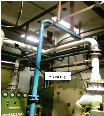
Figure 2: Frosting in suction line.
