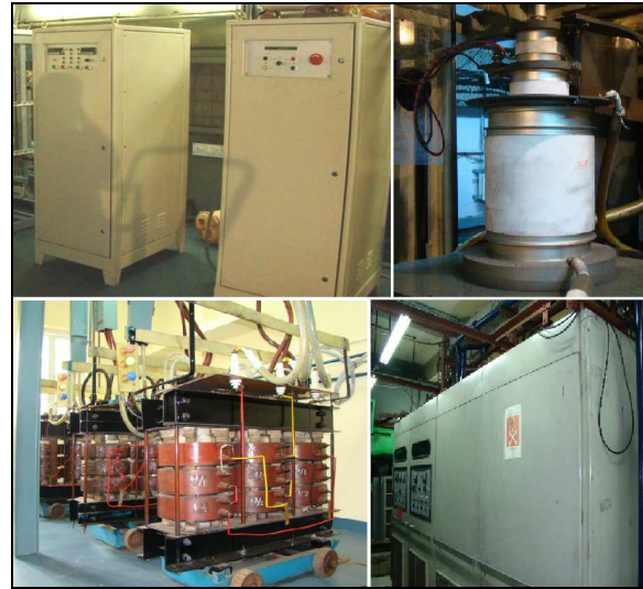
Figure 5: clockwise from left (a) Filament and Screen Power Supply, (b) Anode Series Pass Triode, (c) Transformer Plant Room, (d) Anode Power Supply.
